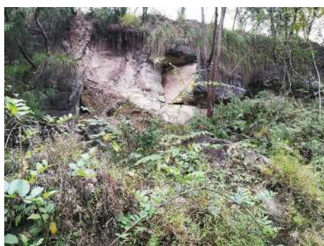
(a) 坡脚局部滑塌
